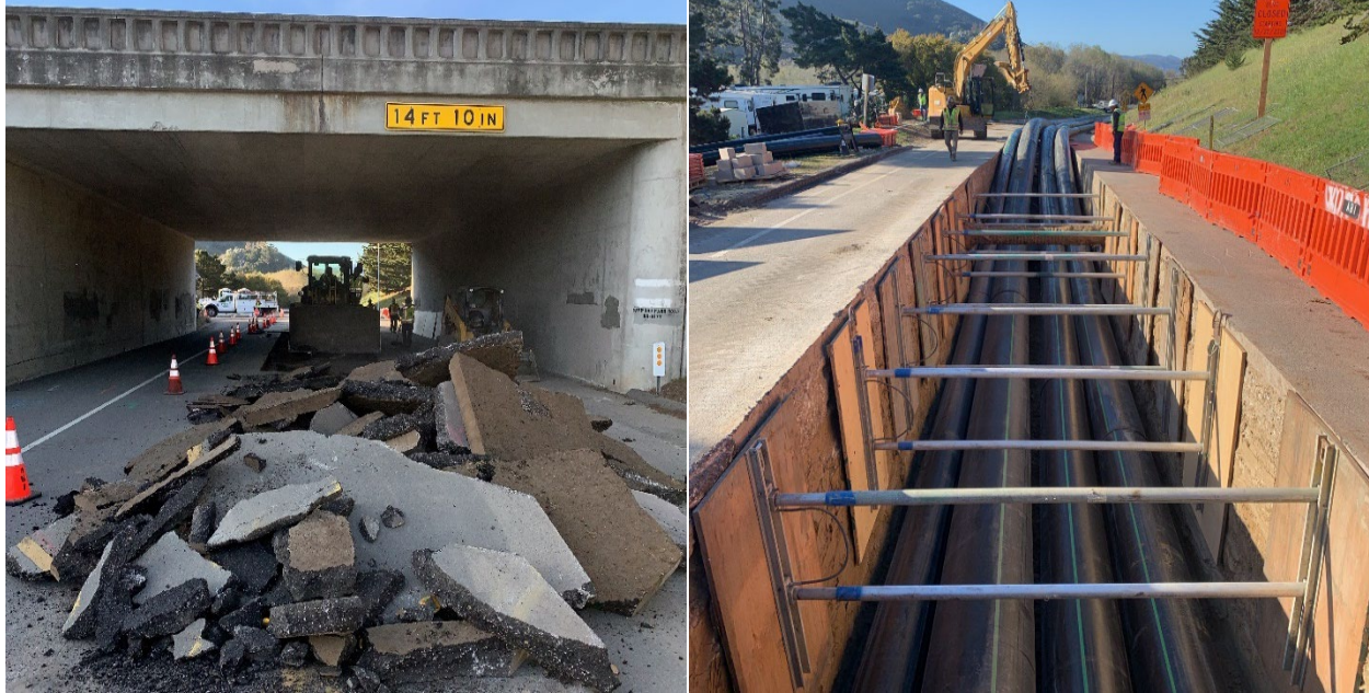
Asphalt removal beneath Highway 1 and Joint Trench on South Bay Boulevard near Highway 1
