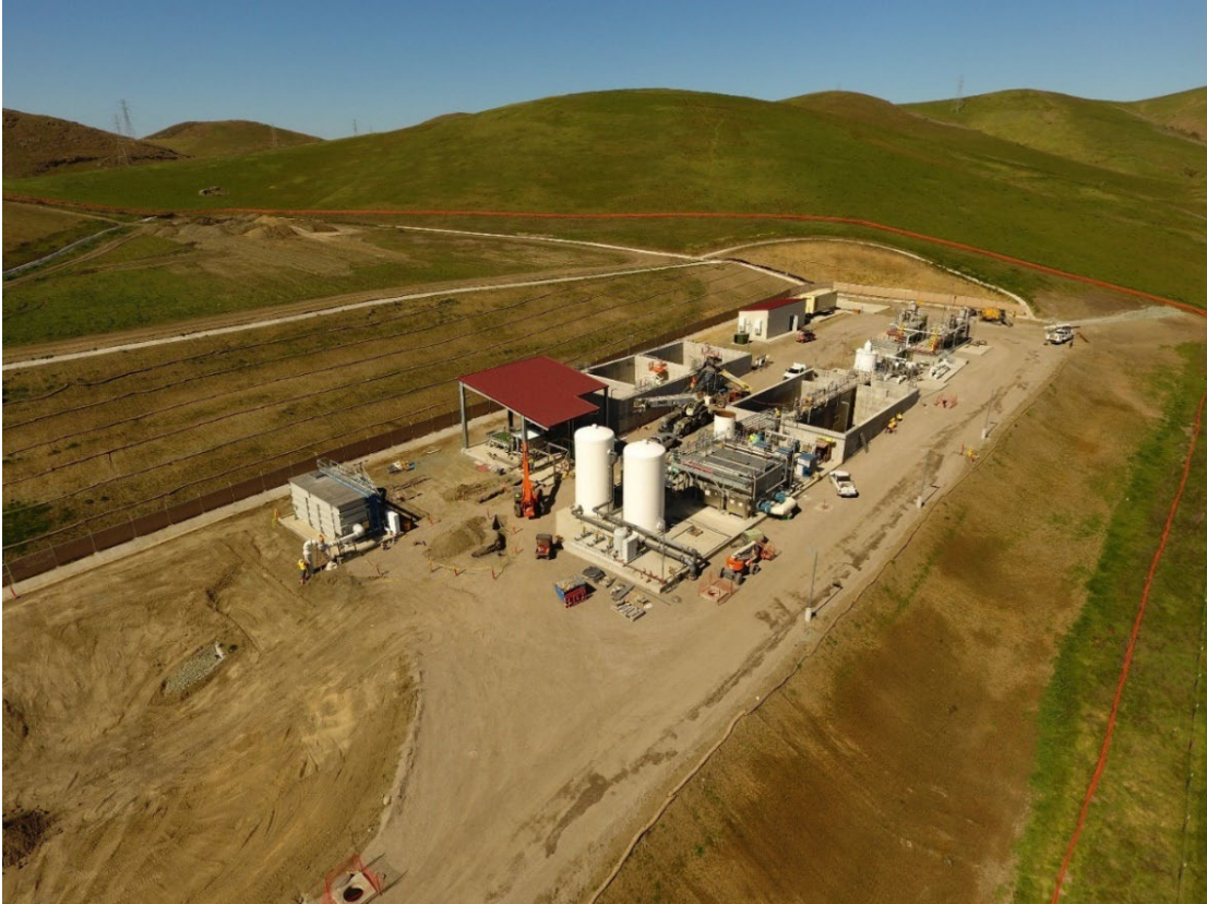
Aerial Capture of Headworks, BNR, MBR, Sludge Holding Tanks, SAFE System on February 28, 2022
