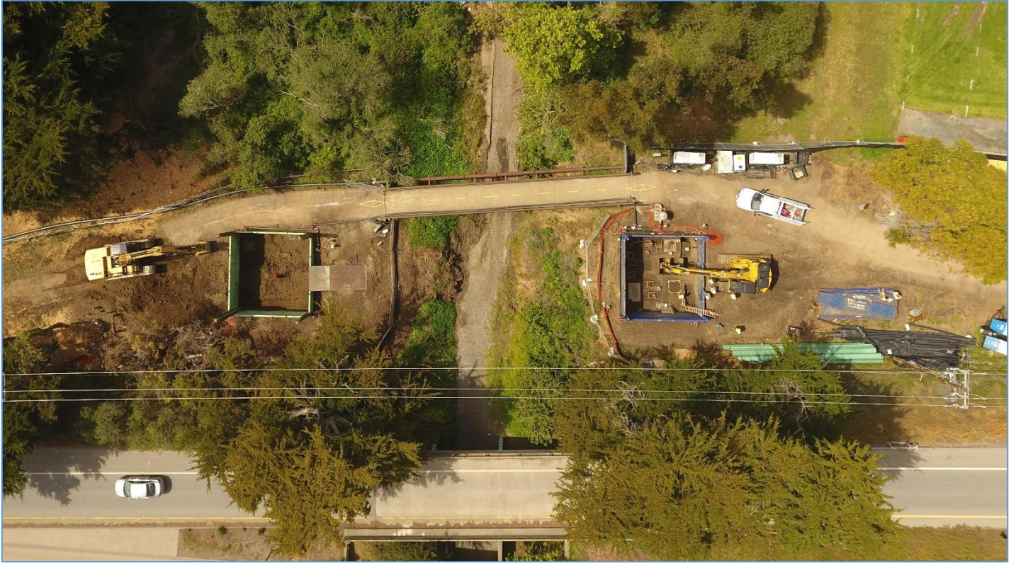
March 31, 2022 – Segments 2 & 3 (Excavating and shoring Utility Bridge abutments at Morro Creek crossing)
