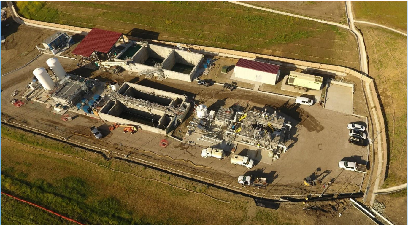
March 31, 2022 – Looking West – North Site (Headworks, BNR, MBR, RWPS, SAFE, Residuals Area, SHT, Elect Bldg) ... Note on-going grassland regrowth, installed curbs, and perimeter fencing, wet testing in progress ...
