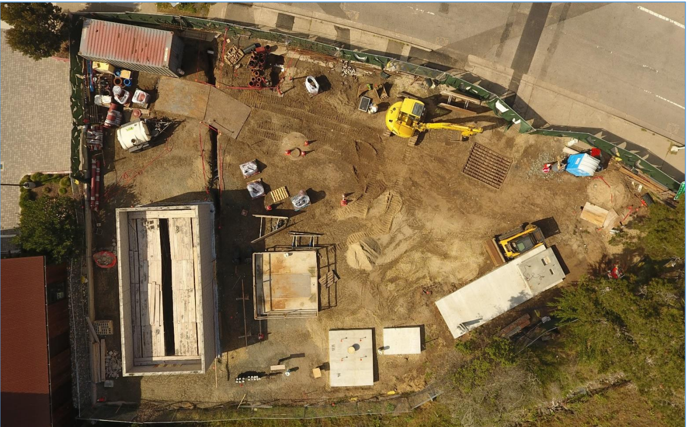
March 31, 2022 – Pump Station B (Elect Bldg masonry, slabs placed for Surge Tank, Odor Control, Generator )
