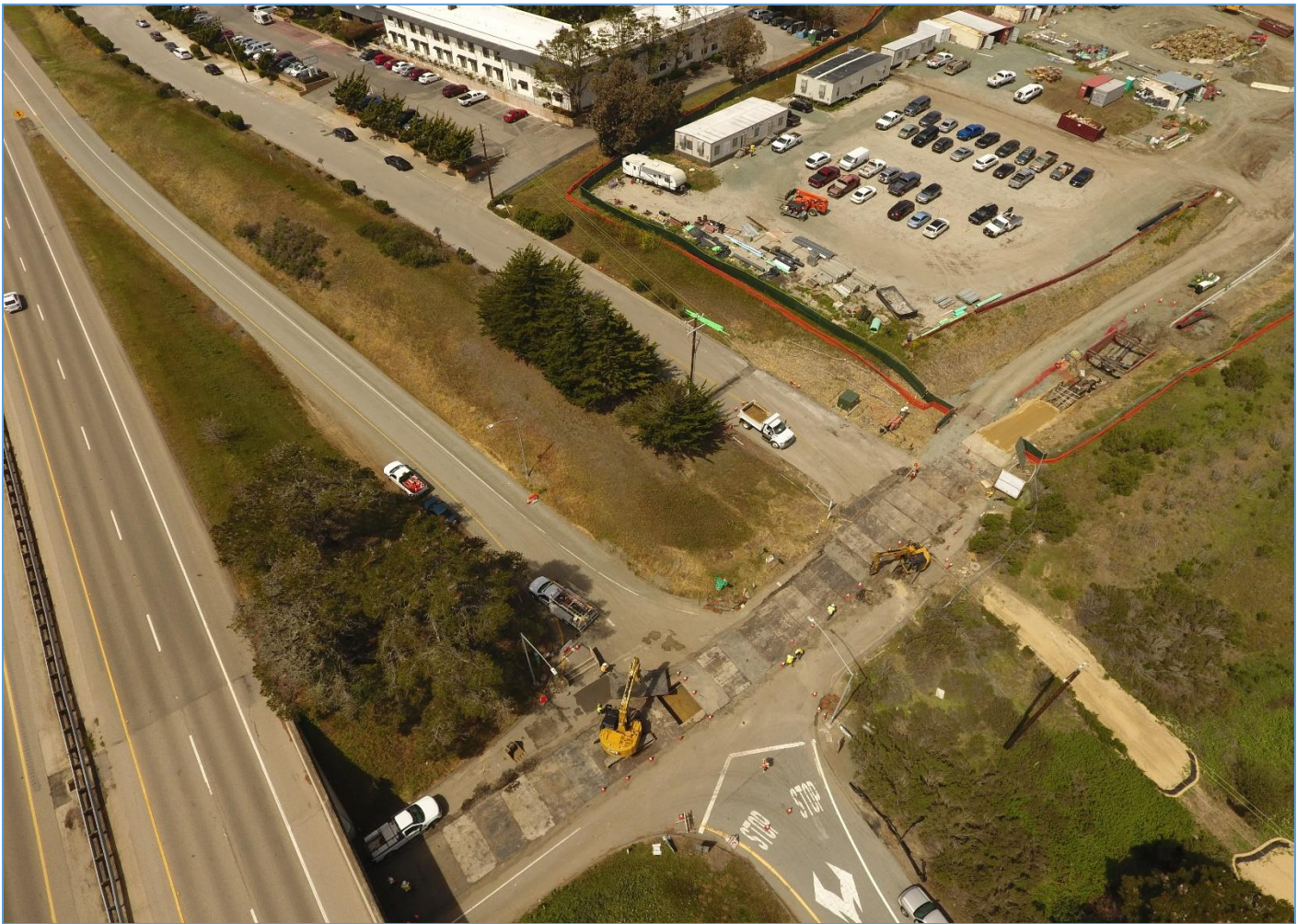
March 31, 2022 – Segment 8 (South Bay Blvd – Quintana to WRF) – Trenching connection to WRF site
