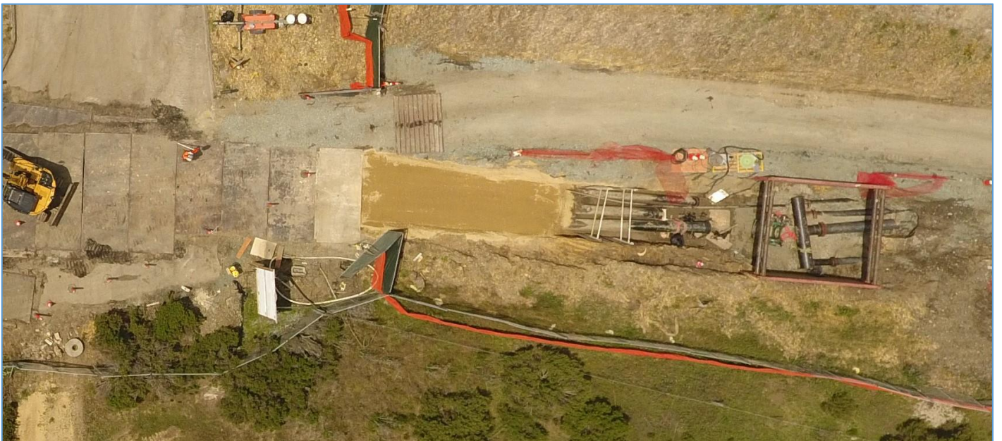
March 31, 2022 – Segment 8 (South Bay Blvd – Quintana to WRF) – Point of connection between projects (Anvil > FBV)
