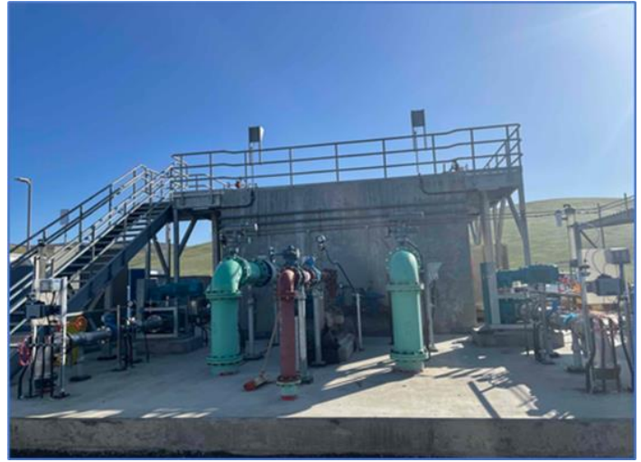
March 31, 2022 – MBR Facility
