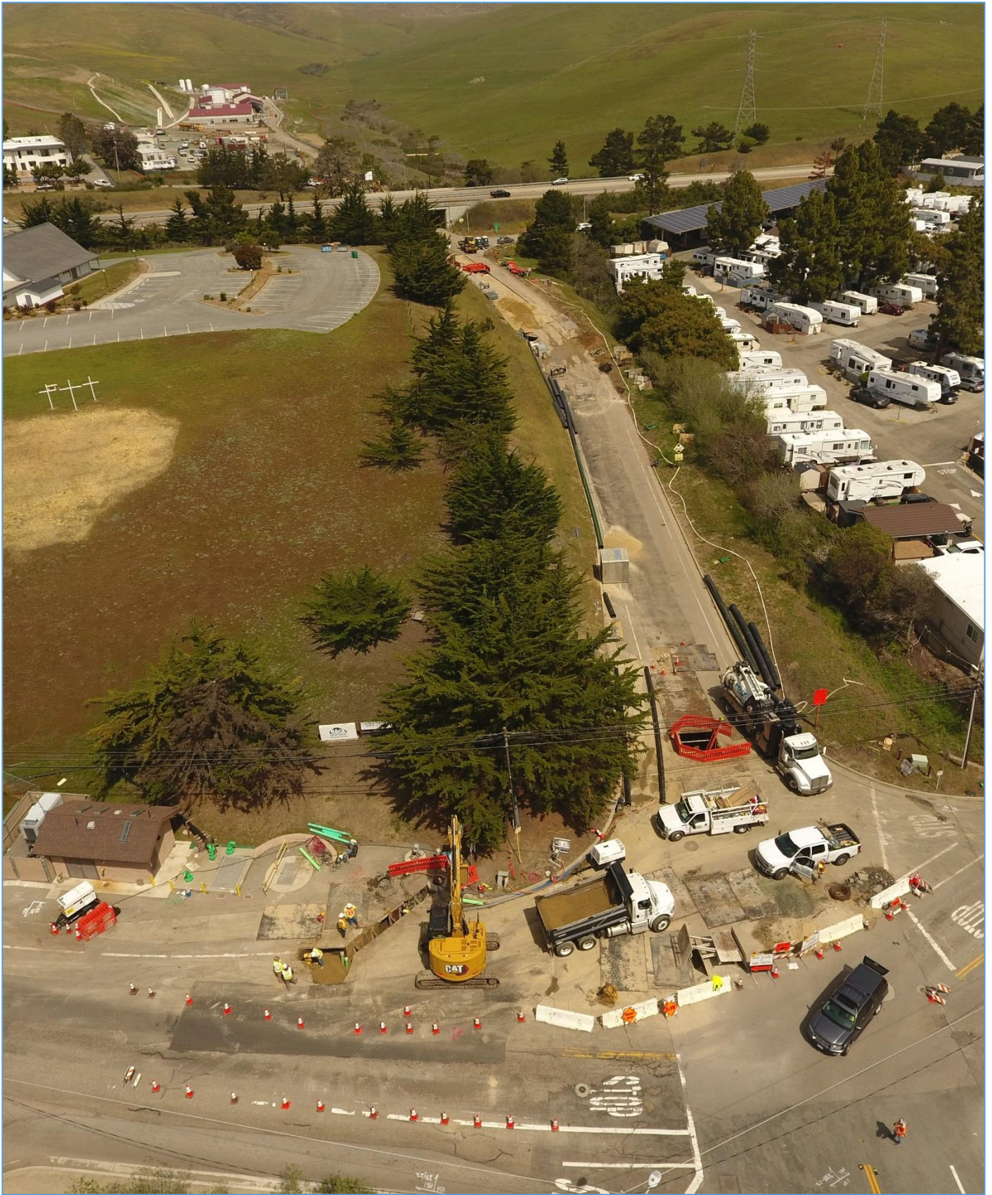
March 31, 2022 – Segment 8 (South Bay Blvd – Quintana to WRF) - Looking north from LS-3 to new WRF site, upper left
