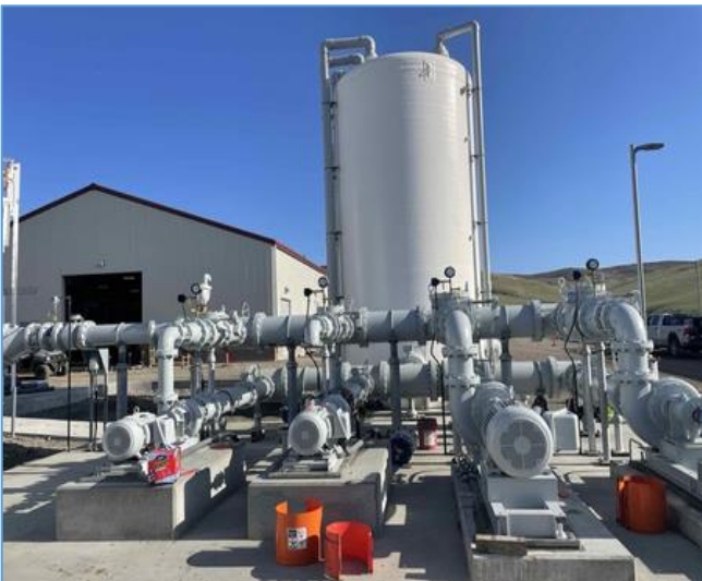
March 31, 2022 – Outfall Pumps
