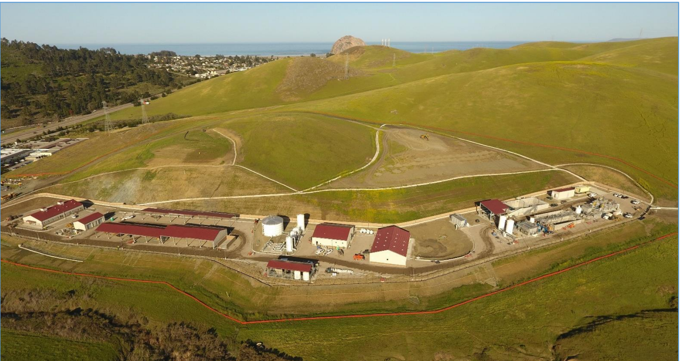
March 31, 2022 – Looking West – Entire Site (Ops Bldg, Maint Bldg, RO/UV Bldg, MBR Plant, Headworks, Etc.)
