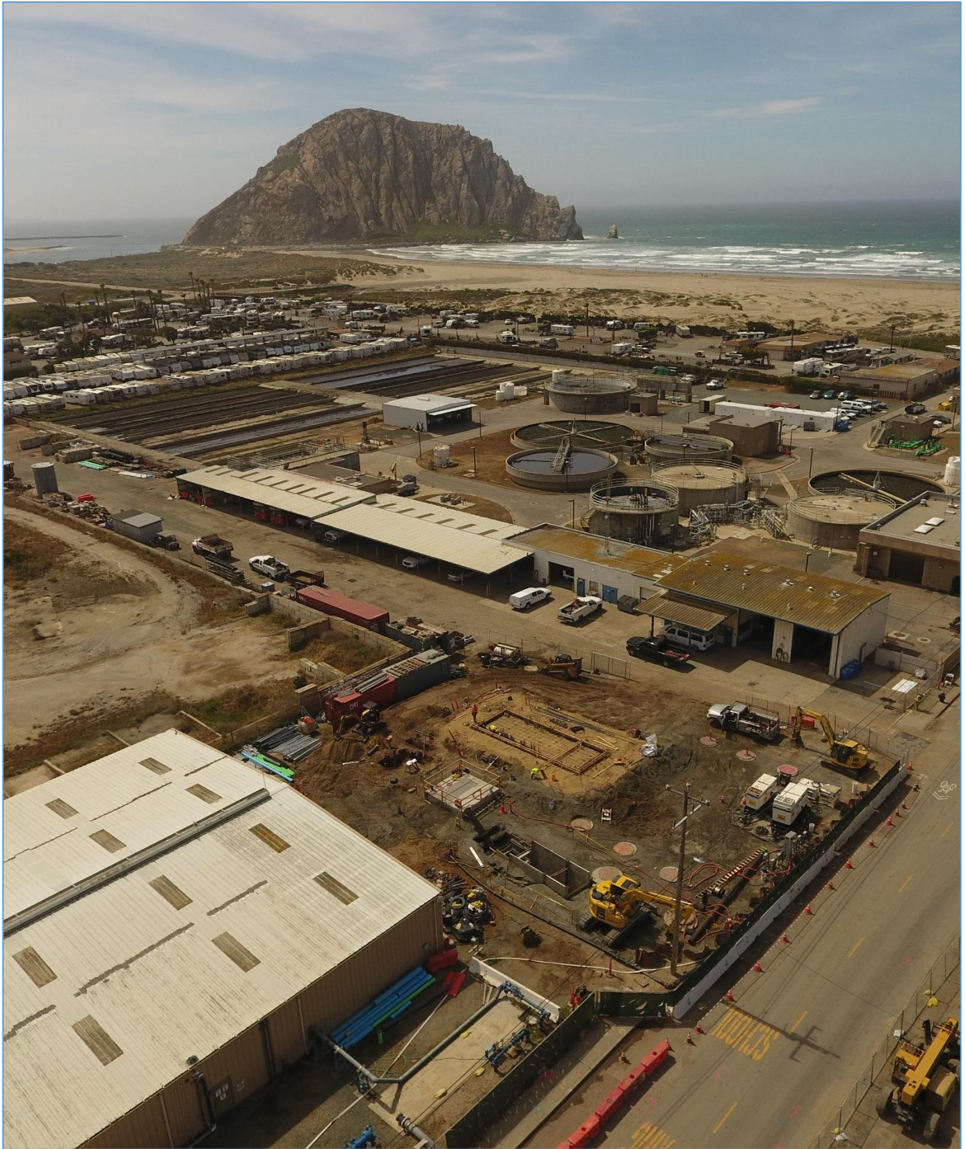
March 31, 2022 – Pump Station A (Emergency Storage Tanks backfilled / Electrical Bldg Slab-on-Grade in progress)
