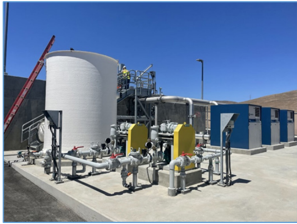
June 30, 2022 – WAS/SCUM Pump Station
