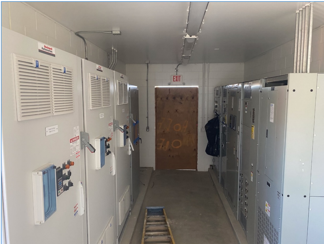
June 30, 2022 – Pump Station A - Electrical Building and Equipment (Green Tagged by PG&E)
