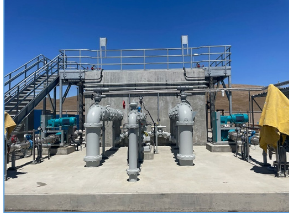
June 30, 2022 – MBR Facility
