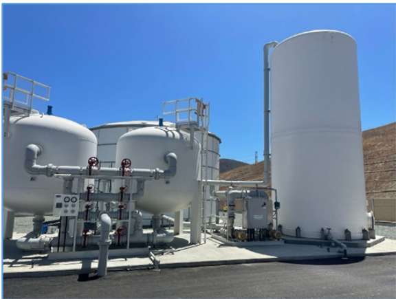
June 30, 2022 – Calcite Treatment Facility
