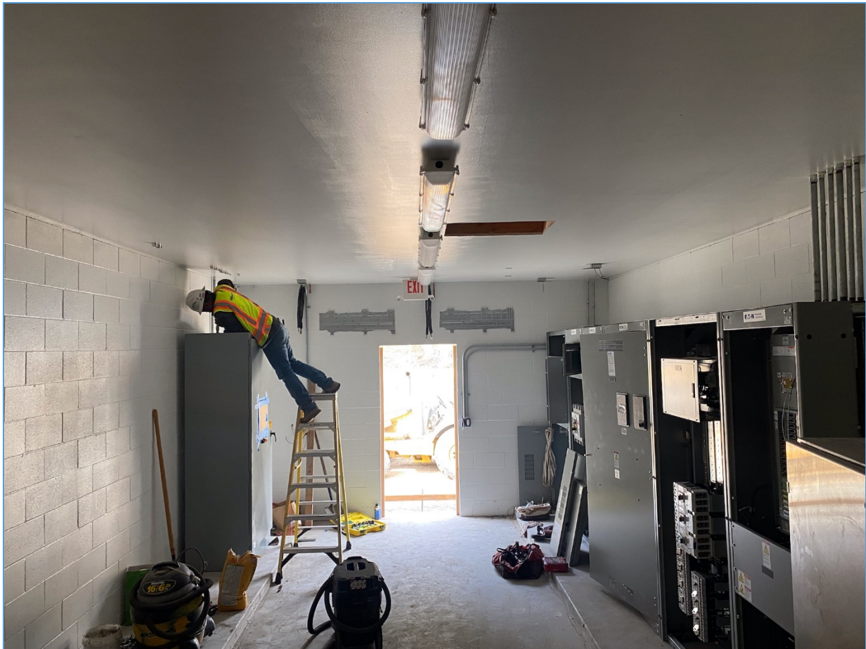
June 30, 2022 – Pump Station B - Electrical Building and Equipment (Green Tagged by PG&E)
