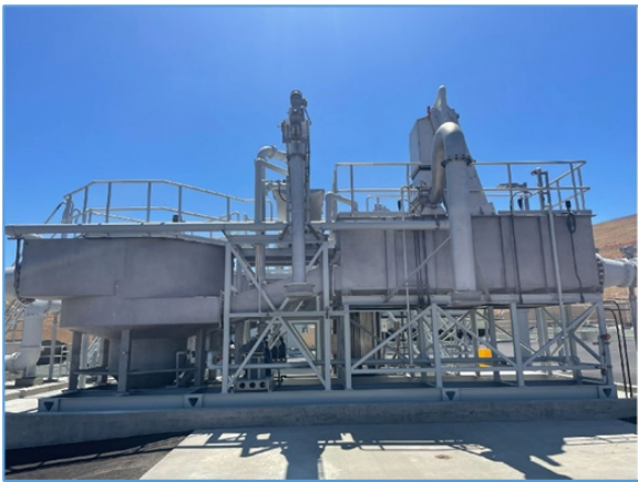
June 30, 2022 – Headworks Skids
