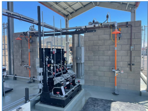
June 30, 2022 – Chemical Feed Facility
