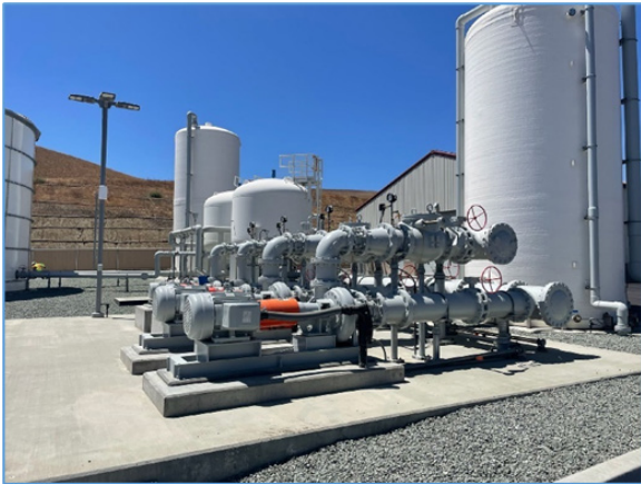
March 31, 2022 – Outfall Pump
