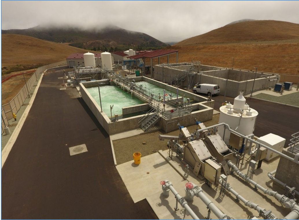
September 27, 2022 – Looking south (Fine Screens and Odor Control, BNR basin clean water testing)
