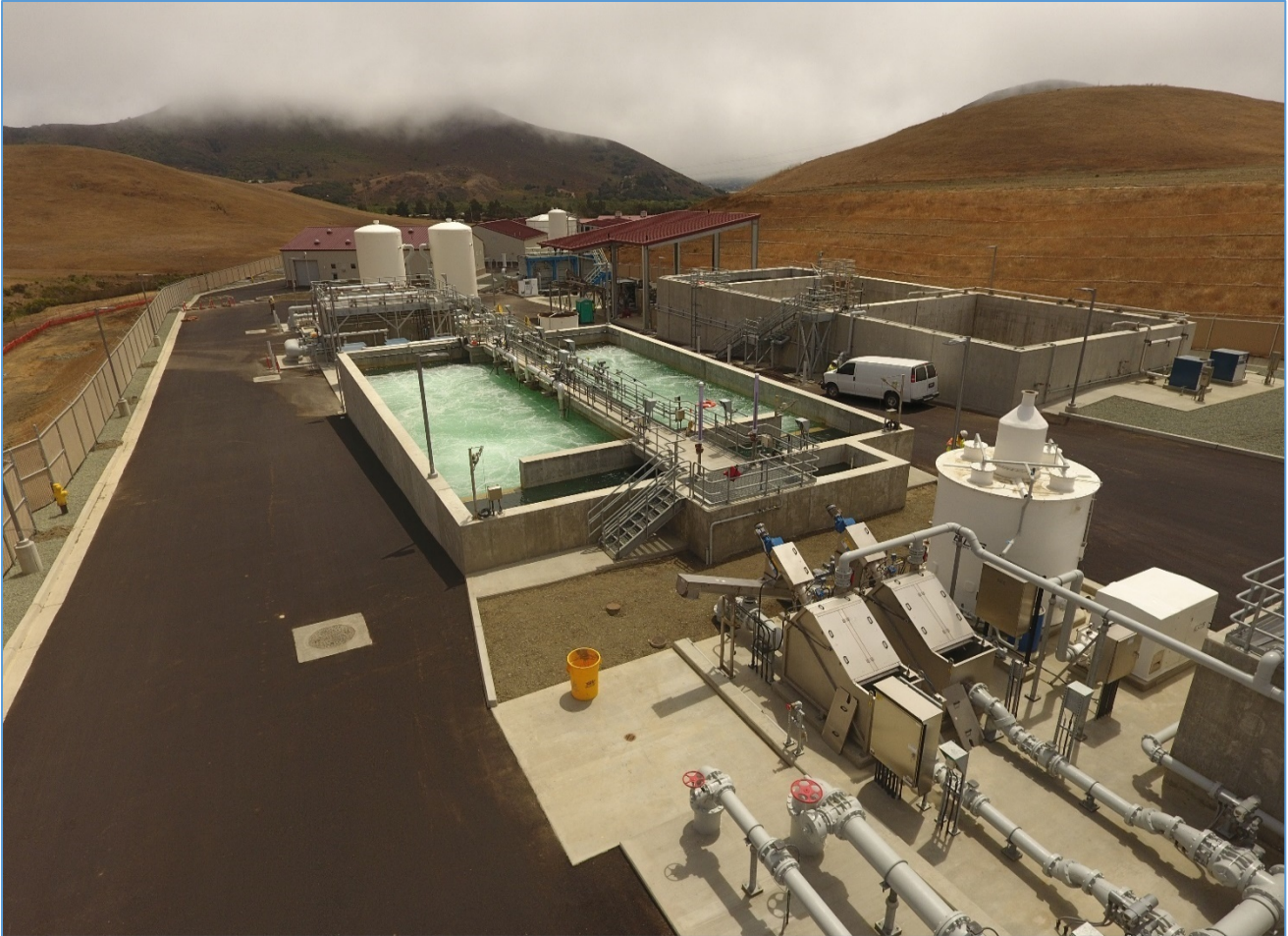
September 27, 2022 – Looking South (Fine Screens and Odor Control Lower Right , BNR Basin Clean Water Testing Center)
