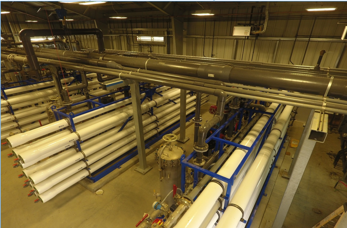
September 27, 2022 – RO/UV Building, Looking at RO Units
