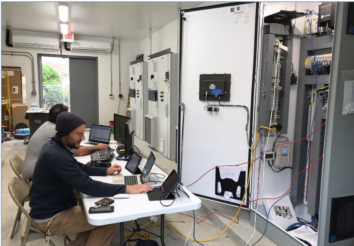
September 30, 2022 – City Staff Setting-up and Testing Pump Station B Programmable Logic Controller.
