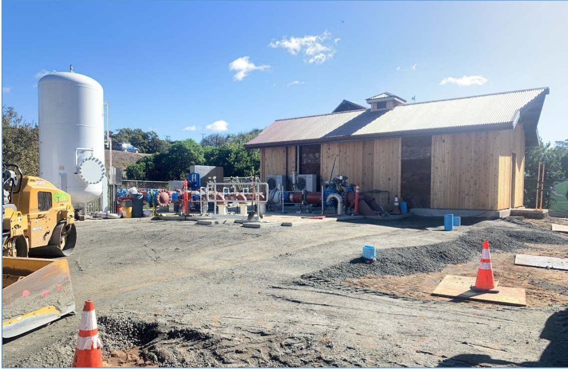
Nov 2022 – Pump Station B Electrical Building, Surge Tank, Discharge Piping, and Site Grading.
