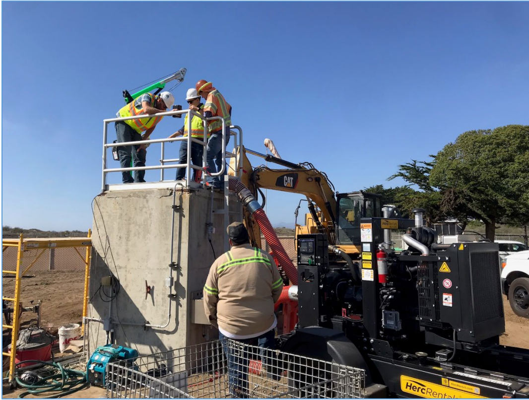
October 2022 – Clean Water Flushing New Brine Line at the City’s Existing Ocean Outfall Box.
