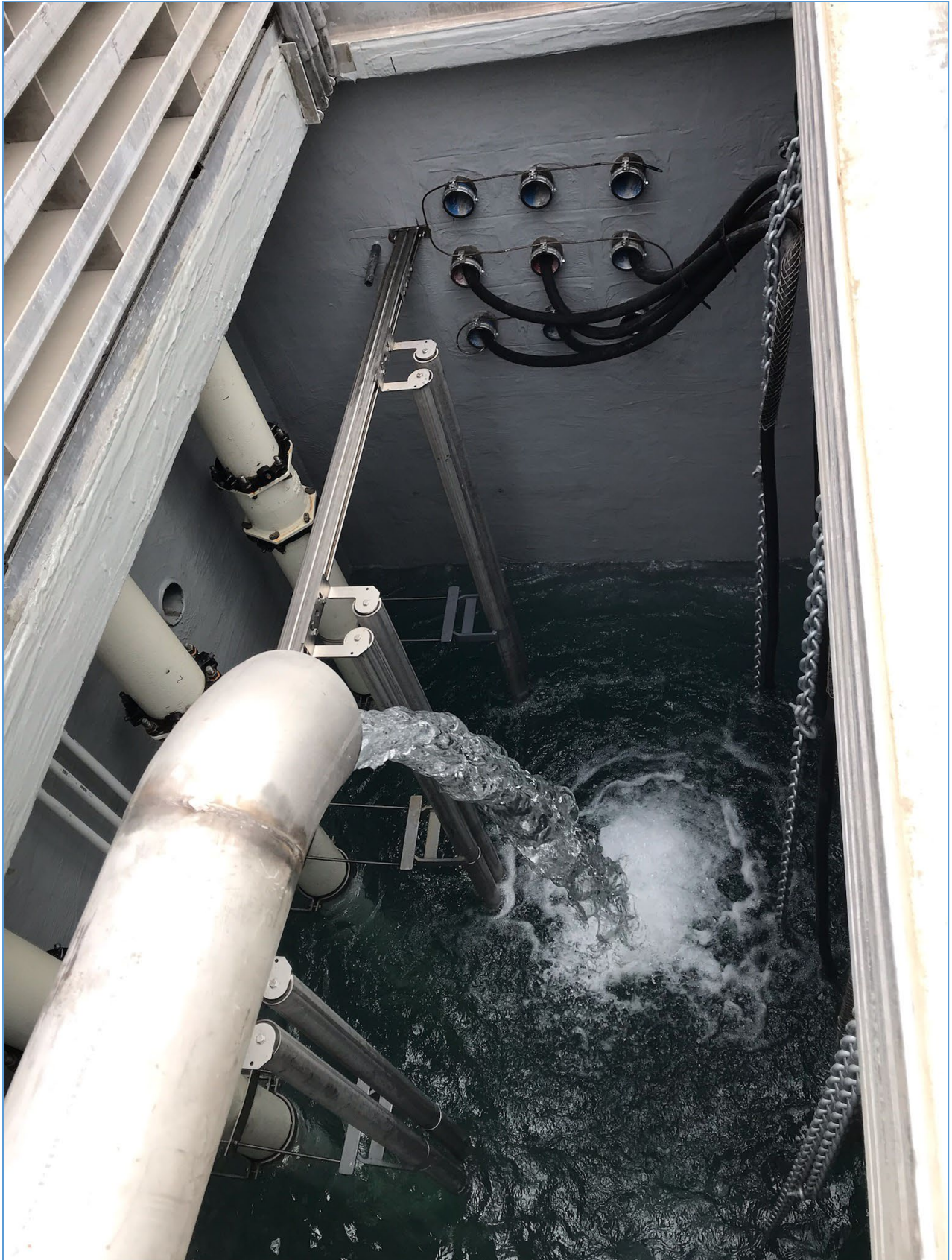
October 2022 – Clean Water Testing and Flushing at Pump Station B Wet Well.
