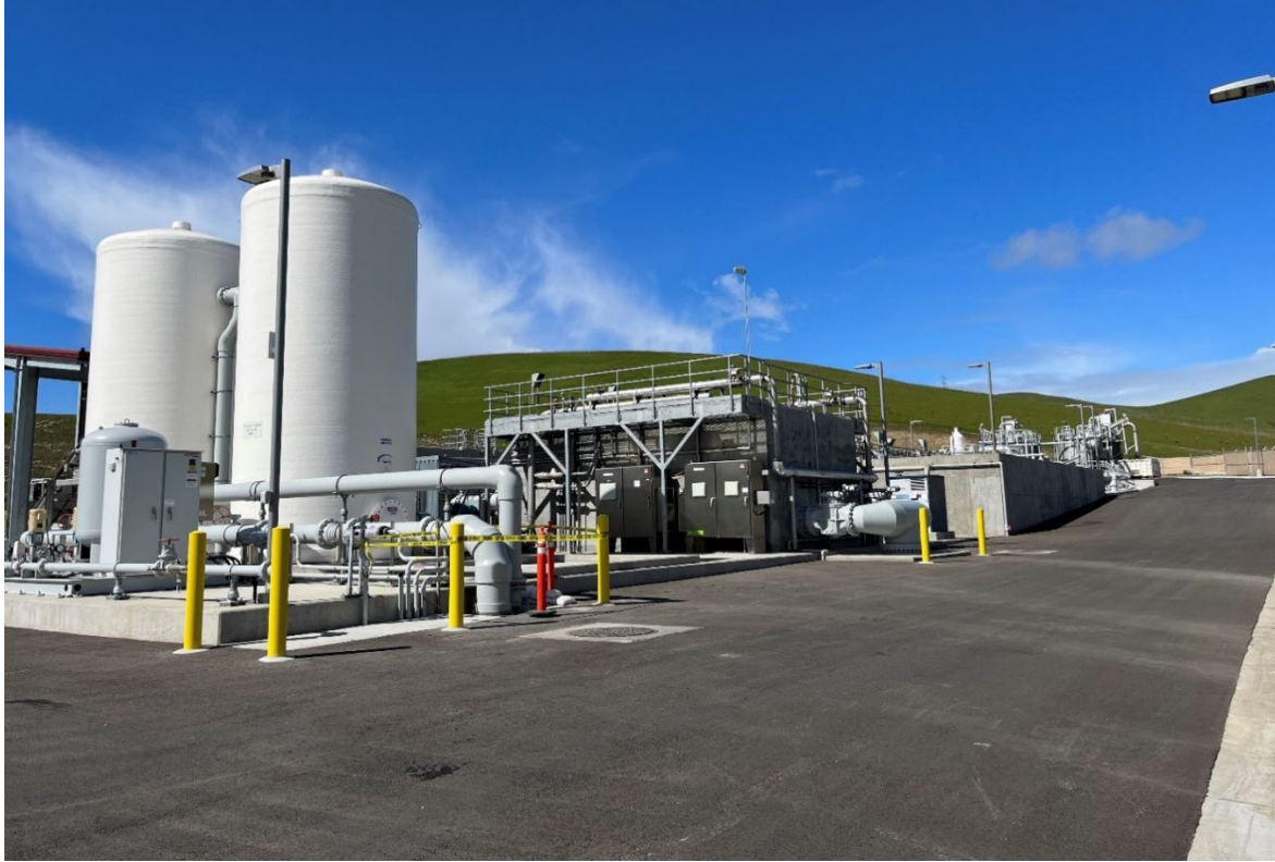
February 23, 2023 – Completed and Operational Headworks and Fine Screens
