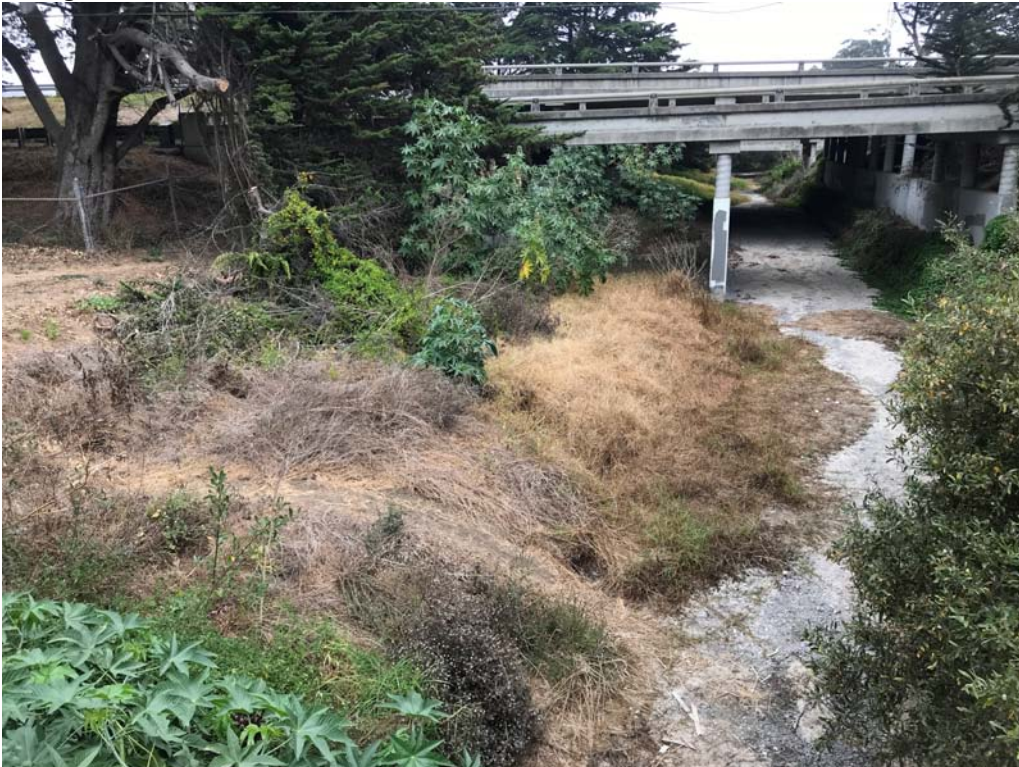
Photo 4. View of Morro Creek and pipe bridge location in the fall 2019 showing dry channel with no aquatic habitat. Abutments will be constructed outside the top of bank on each side of creek and the pipes dropped in place using a crane.
